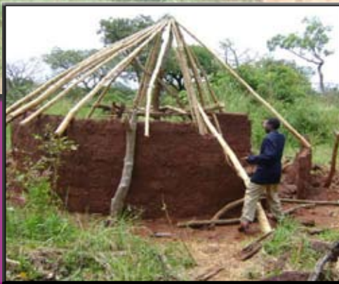
Rev. Alfred Komakech inspect and house being constructed for him at the Parish headquarters Lakwana.
